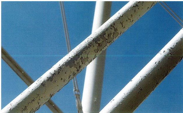
Corrosion on Diagonal Bracing - College Tank
