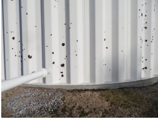
Corrosion on Vine Street Tank Exterior
