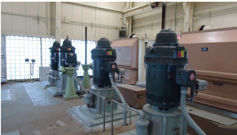
Vertical Turbine Pumps and Travelling Screens @ Raw Water Intake
