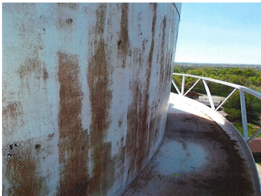
Corrosion on the Frontier Tank
