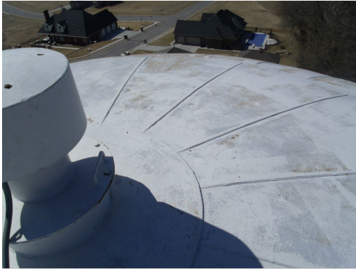
Loss of Coating on the Roof of the Green River Road Tank
