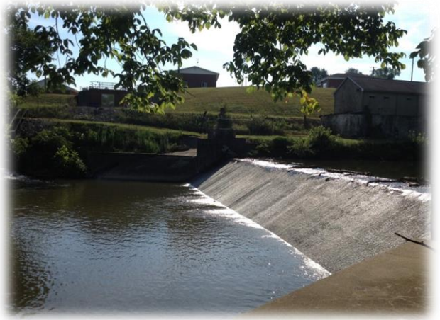
View of the Dam at Mt. Sterling Water & Sewer Water Treatment Plant
