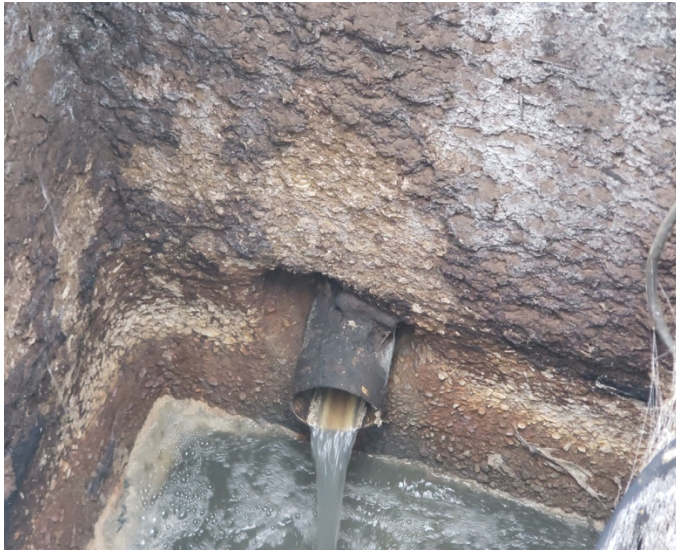
Sewer Pump Station Below Old Dairy Queen Building
