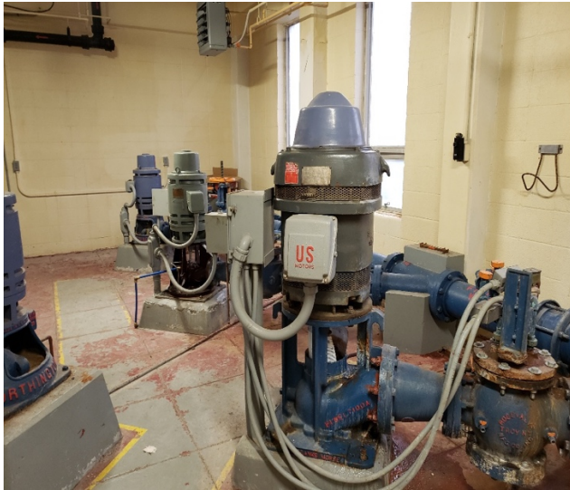
High Service Pumps
